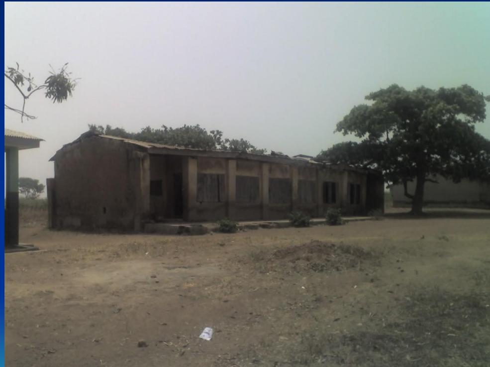
Unsafe classroom building
