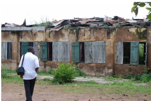
This is current uninhabitable primary school building block.
